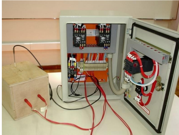
Figure 4 – Temperature Control System
