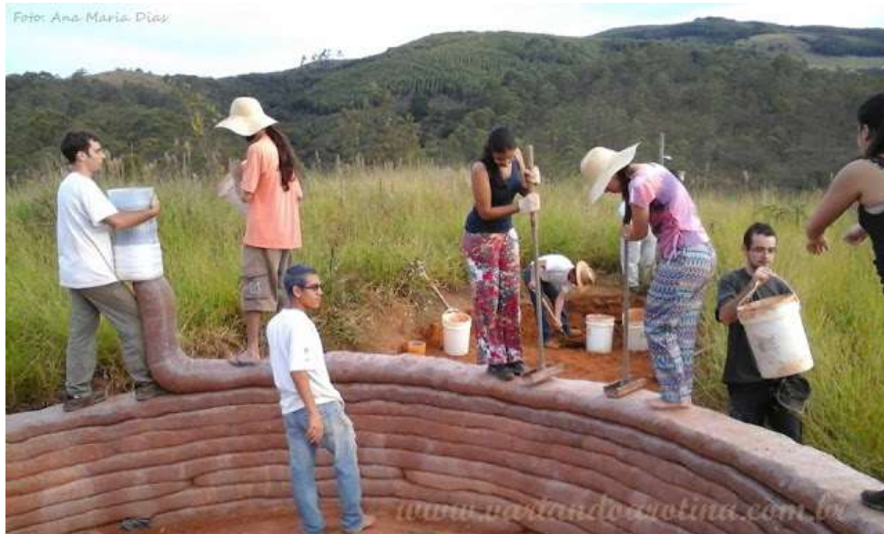
Figure 2 – Construction with hyperadobe - bag filling (workers on the left) and on-site compaction (on the right).
